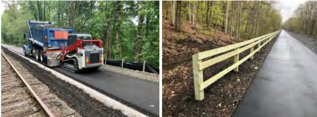
The Maybrook Trail, Putnam County, NY, (part of the EST under construction in 2020), with approximately 23 miles of shared-use pedestrian and bicycle rail trail alongside tracks owned by Metro-North Railroad (Photo: https://maybrooktrailerway.org/ )
