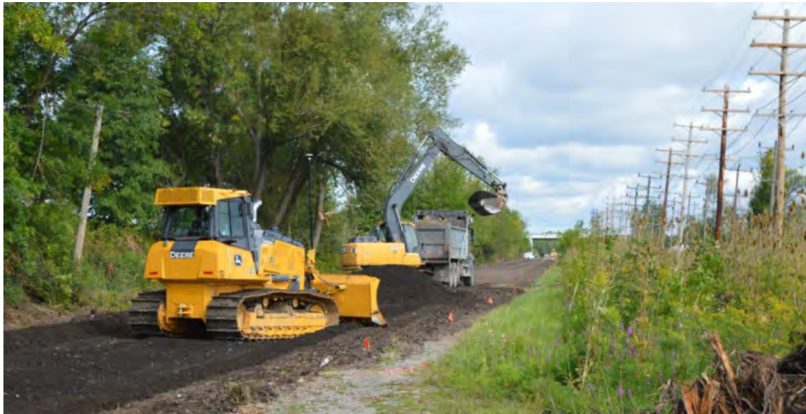
The 3.9-mile Tonawanda Rails-to-Trails, shown here under construction, is comprised of two segments on a former railroad bed (Photo: Buffalo Rising)
