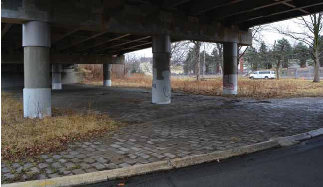
Photograph 14. Pylons and concrete-block paved surface beneath the Robert Moses Parkway in Survey Area 5, facing northeast (Panamerican 2016).
