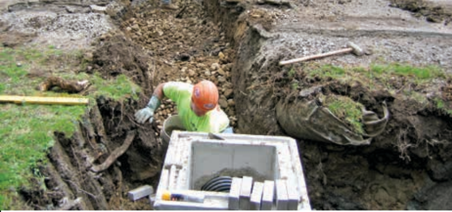
Replacing the culvert at Letchworth State Park is an example of the countless projects to maintain unseen but essential infrastructure throughout the park system.
