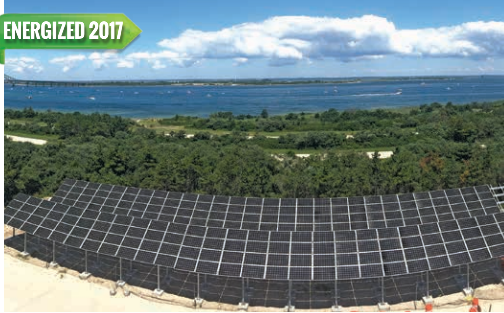
The major solar power system creates enough electricity to serve Robert Moses State Park's 4 million visitors a year and created one of the first energy neutral state parks.
