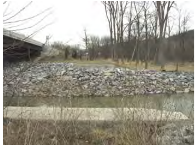
Bridge abutments constructed by NYSDOT for bridge over Cayuga Inlet to Buttermilk Falls State Park
