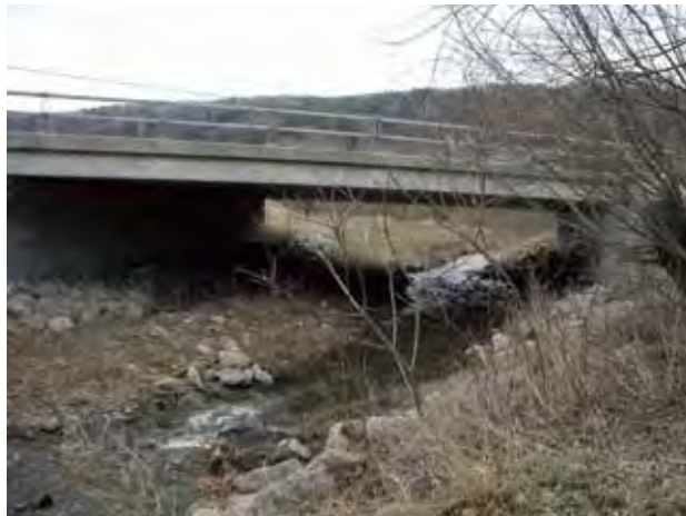
Trail underpass of N. Y. S. Rtes 13/34/96 at Robert H. Treman State Park
