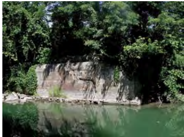
Existing bridge abutment from former lehigh Valley rail crossing of the Cayuga Inlet
