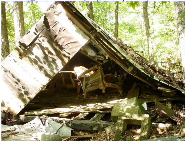
Awosting_PN 9-4-09 collapsing shack-private-public border
