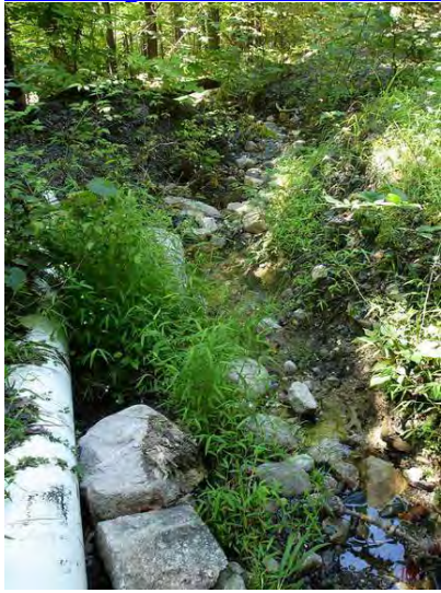
Awosting_PN9 9-2-09 Stream crossing and erosion
