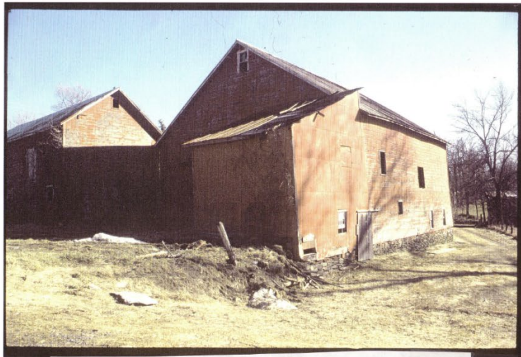
6. Rosedale Dutch barn (Rh-4) looking north Roof damage to the shed addition to The Dutch barn, seen in the center of the photograph, needs repair.
