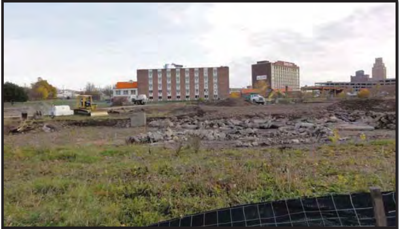
Photograph 1.3. View of construction excavation activity at the southwestern portion of the study area, facing southeast (Panamerican 2014).
