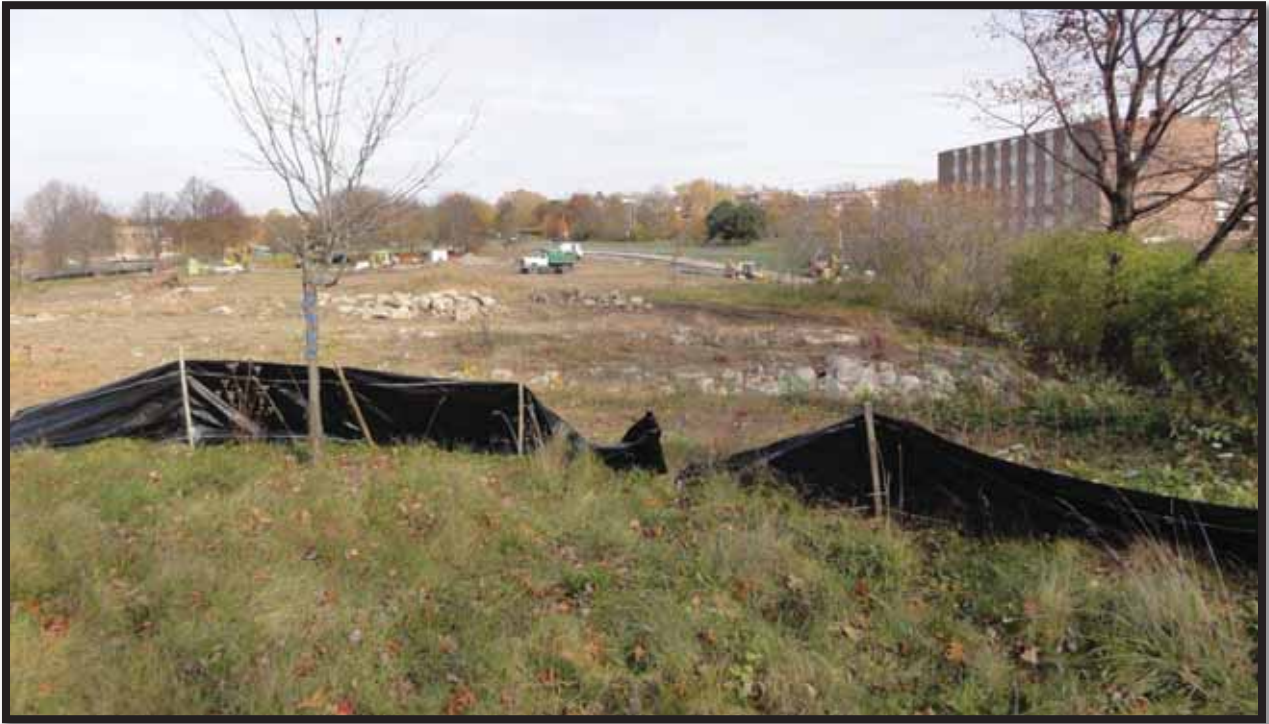
Photograph 1.2. View of construction excavation activity at the southwestern portion of the study area, facing northeast. The activity appears to have uncovered foundations of earlier structures (Panamerican 2014).
