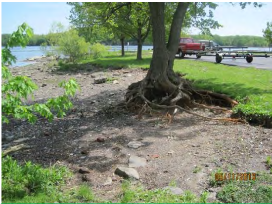
Cossackie boat launch site with heavy erosion, before shoreline restoration
