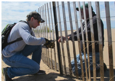
Cam Heasley and Dave Warner install snow fencing at the Sandy Island Beach State Park Bird Sanctuary to protect piping plovers. Photo credit: FORCES NYS OPRHP.
