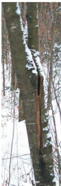
Figure 3.117. If a weak union is also cracked it is very likely to fail.
