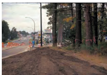
Figures 3.83-3.84. To estimate how much root damage was sustained, determine how much of the Critical Root Radius was disturbed.
