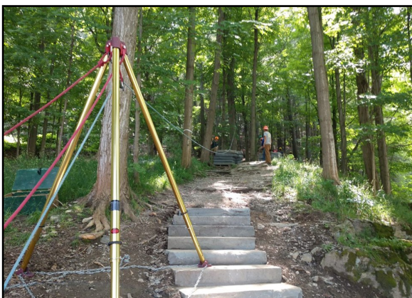
Regional Trail Crew and FORCES Trail Stewards setting up rigging equipment to move stone treads for a staircase at Taughannock Falls SP. Each tread weighs upwards of 300 pounds! Photo: OPRHP
