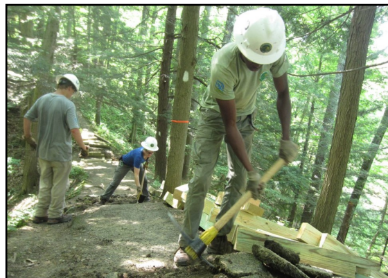
The Excelsior Conservation Corps working with the Finger Lakes Trail Crew and FORCES Stewards to rebuild a timber staircase at Buttermilk Falls State Park. Photo: OPRHP
