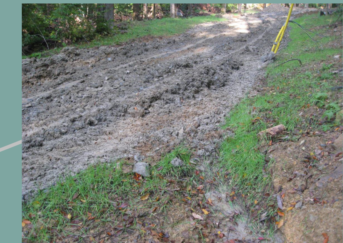
Muddy road with no erosion control.
