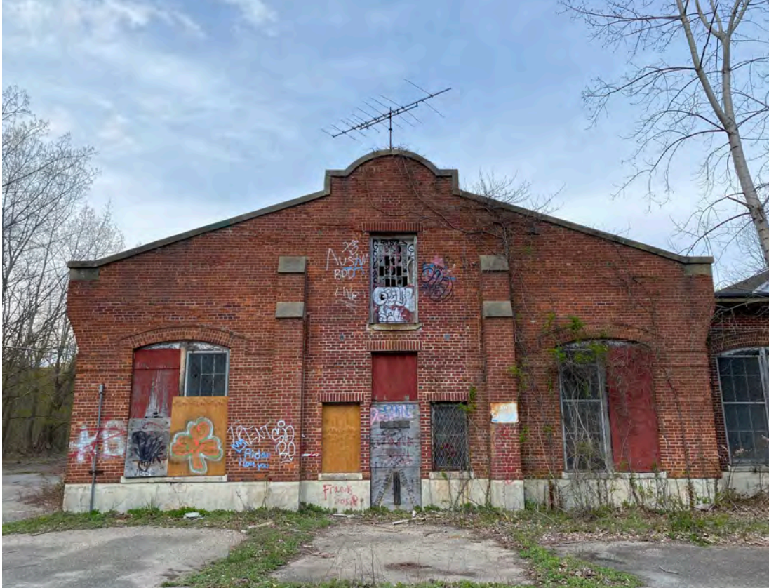
Existing Condition Building 5, the Old Laundry Building, has the structural integrity for reuse.
