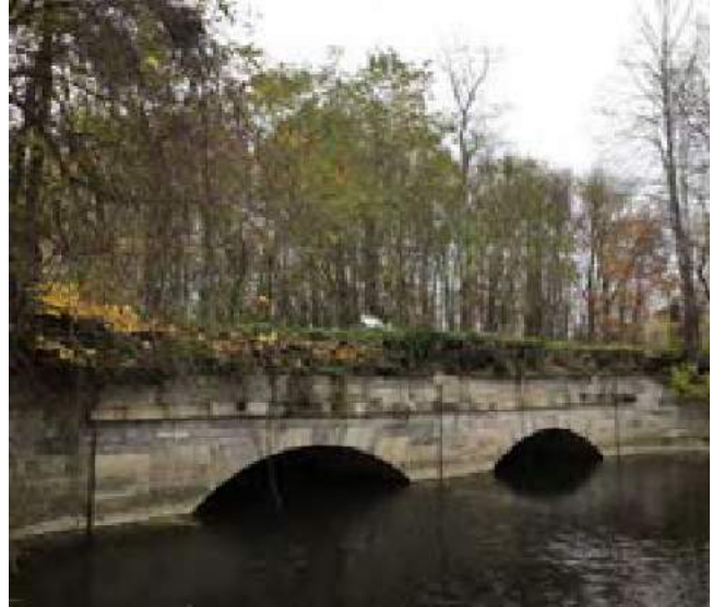
Figure 1: Double arch culvert situated over the Black Creek just south of Rochester.
