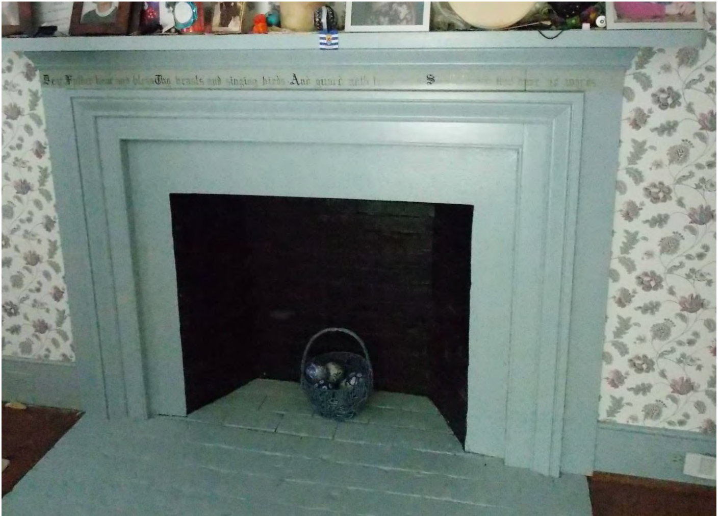
Figure 3. Stenciled fireplace, William W. Gorham House, NYS OPRHP Site visit photograph, July 13, 2022.
