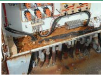
Electrical panel at Clarence Fahnestock State Park
