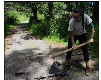
FORCES Steward Alexandra Sakoulas building a trench for a water drain pipe at Glimmerglass State Park.
