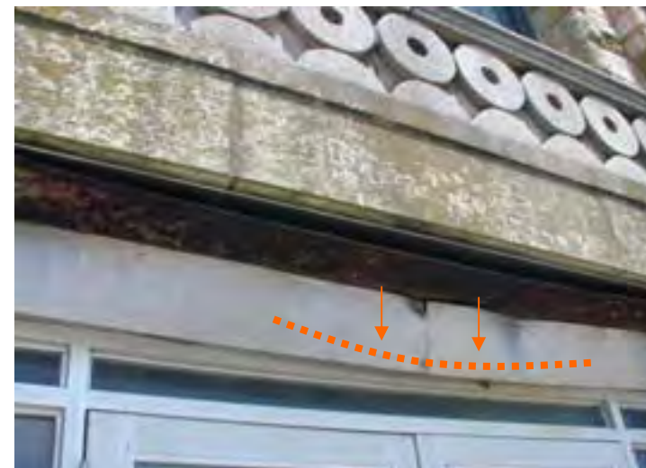
Steel lintel deterioration (South Bldg. South 2009)
