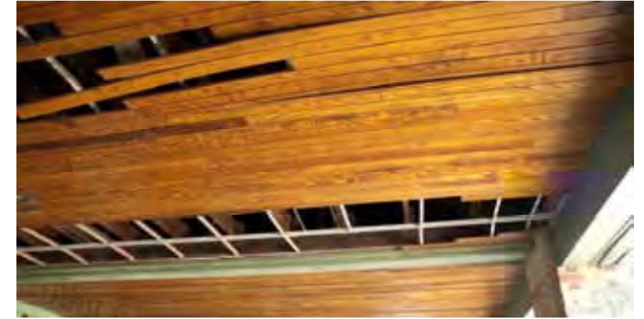
East Bathhouse, Loggia/Lobby 2013—Note: Ceiling failure.
