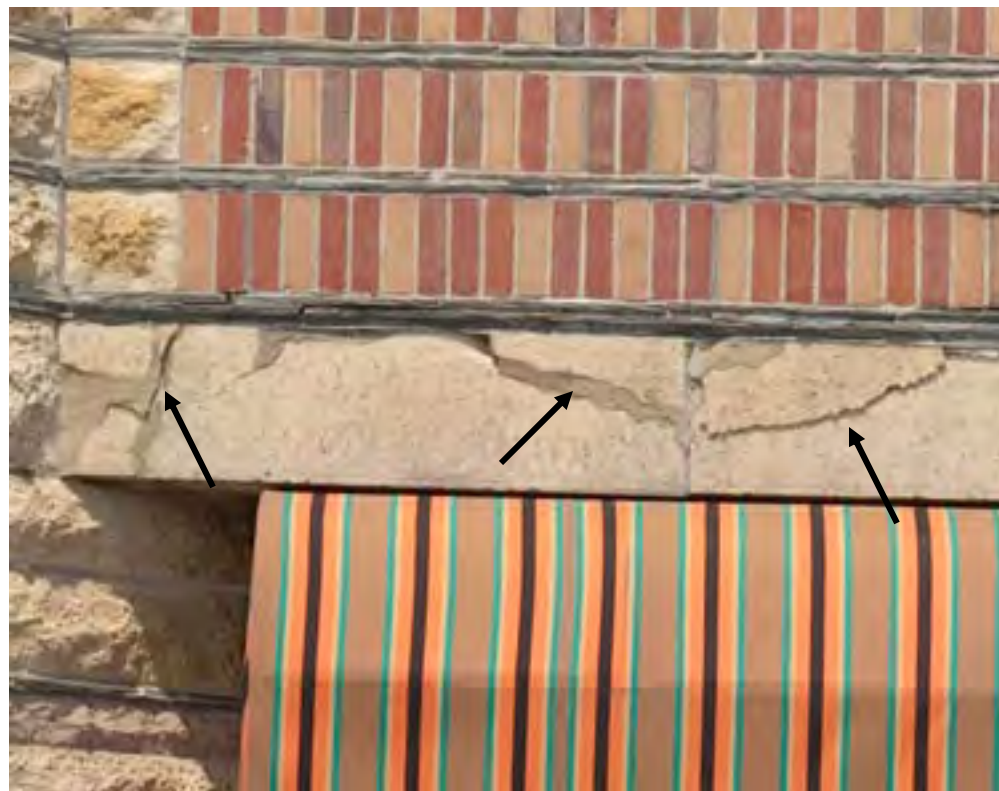
South Façade: Cracking in sandstone lintels.
