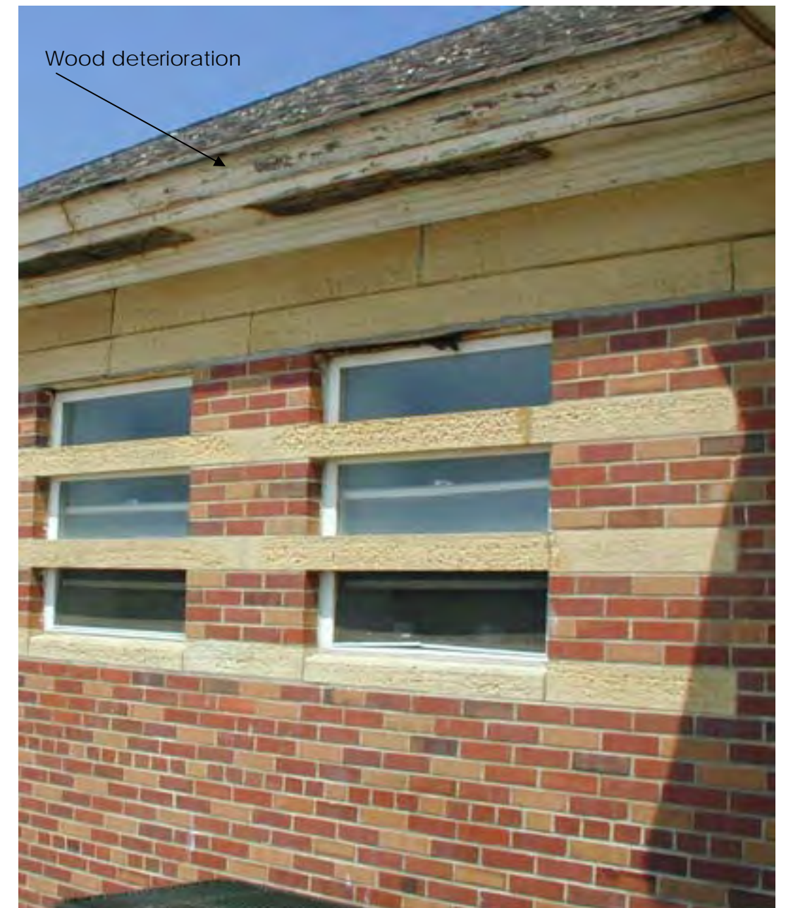
Sandstone & Wood deterioration (south elevation). 2009
