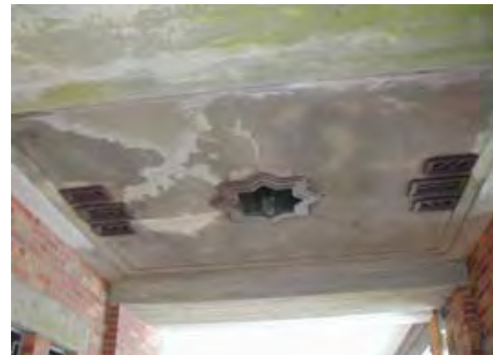
Roof leaks & Deterioration (Loggia. 2009)
