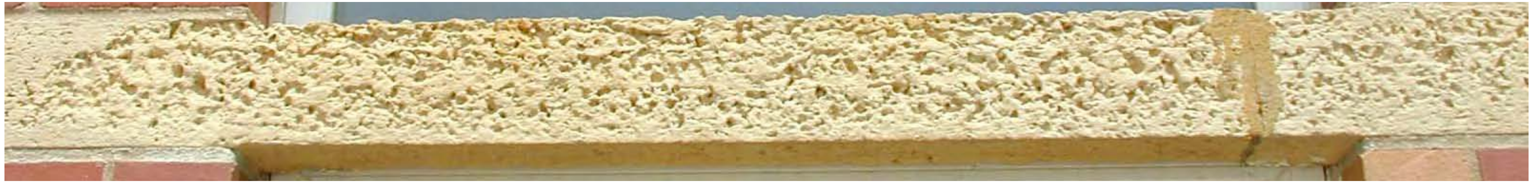
Detail of severe sandstone pitting (south elevation). The surface should be smooth. 2009
