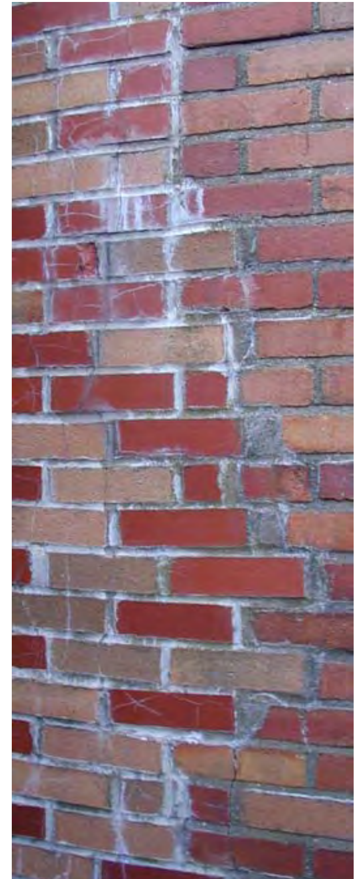
Brick deterioration (Perimeter Wall 2009)
