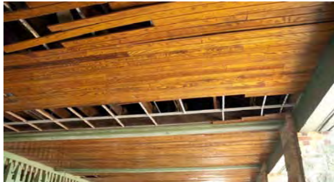
North building ceiling deterioration (2013)
