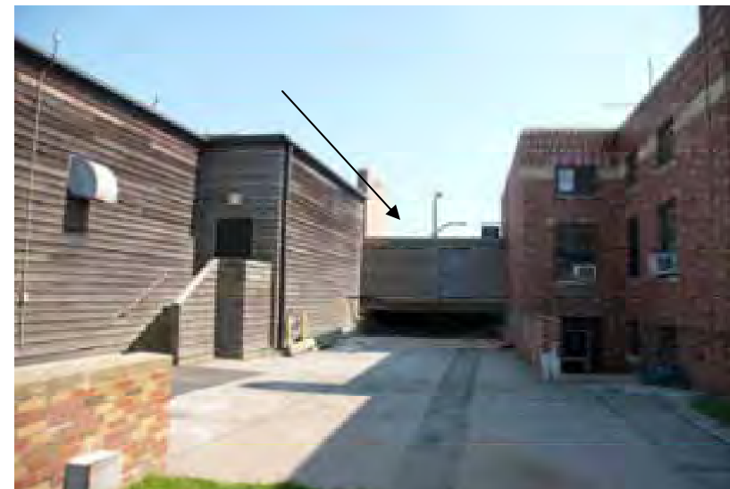
Alley between Administration Building and Boardwalk Café. Note the area is shielded from the boardwalk by the wood
