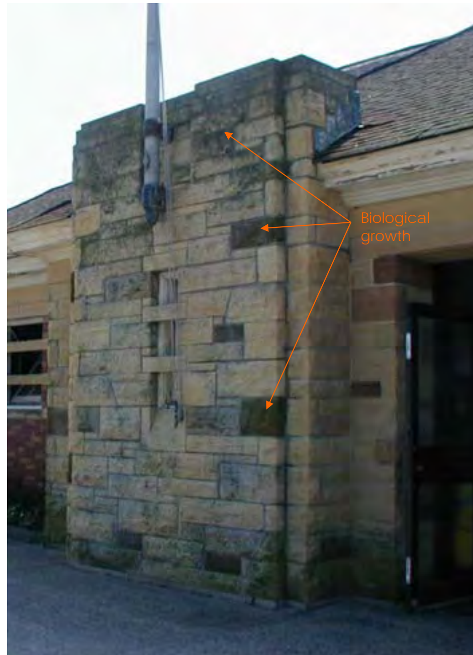
Biological growth— sandstone towers (north elevation). 2009
