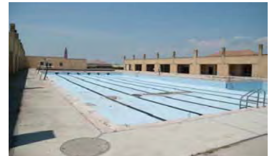
Deterioration of pool lining due to disuse (2013)
