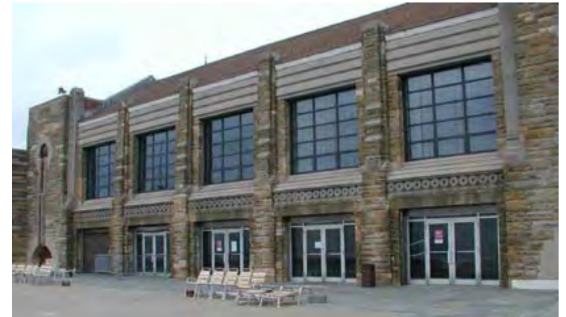
West Bathhouse, South Elevation 2009. Note: collapse of lintels over doors.
