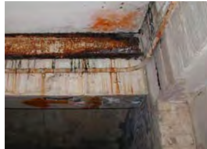
Structural Steel Deterioration (North Bldg. 2009)
