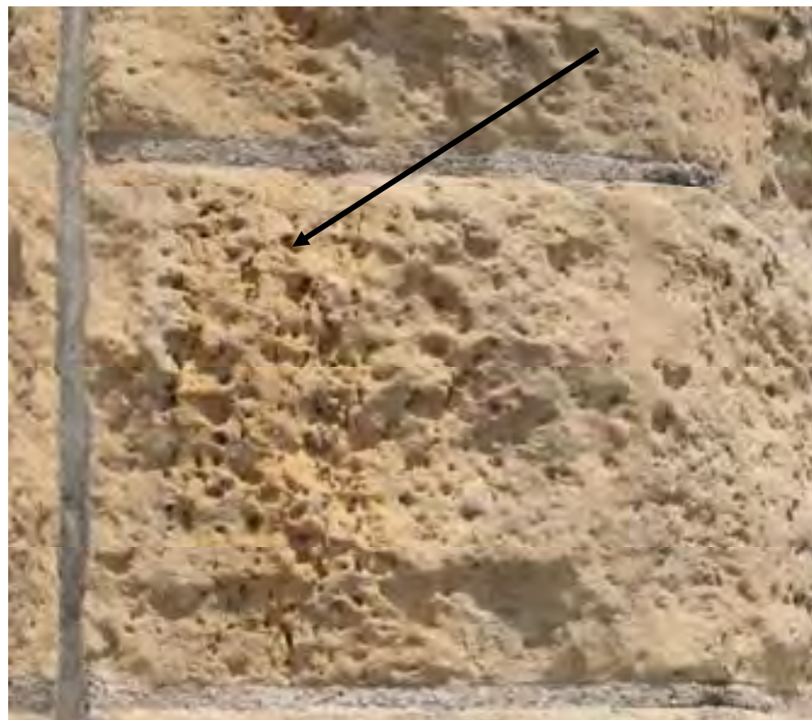
South Façade: Sandstone pitting—typical condition.
