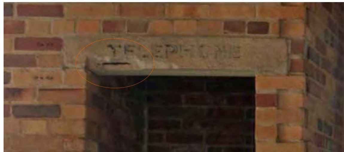
North building concrete deterioration (2013)
