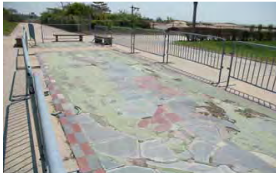
Deterioration of Central Mall Mosaics.
