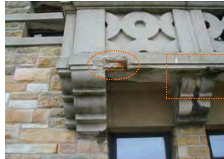
Cast stone Deterioration (South Bldg. 2009)
