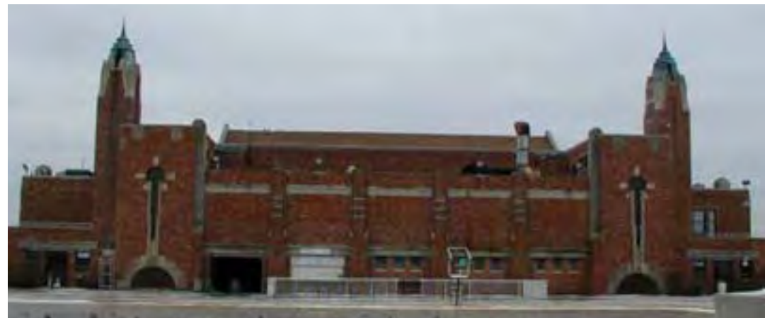
West Bathhouse, South Elevation of Courtyard 2009. Note: infill of ground floor bays and second story windows.
