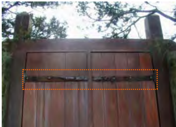
Wrought Iron Deterioration (Perimeter Wall. 2009)
