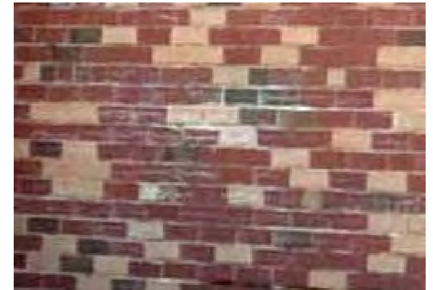
Brick Screen wall—deterioration (2013) Bad picture to be replaced
