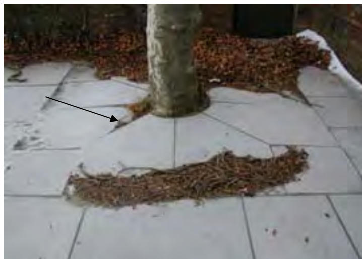
Pavement displacement (Pool deck. 2009)
