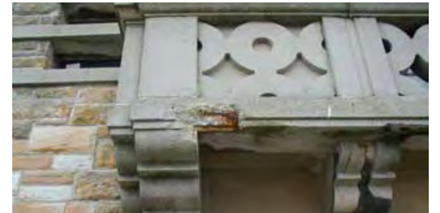
West Bathhouse, South Elevation 2009—Note: Cast Stone failure.
