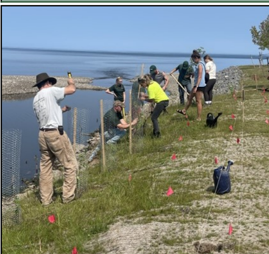
Park staff and FORCES members installing native trees along the shoreline of Grindstone Creek as part of a shoreline restoration effort. The goal of the project is to reduce erosion in the area. Photo: OPRHP
