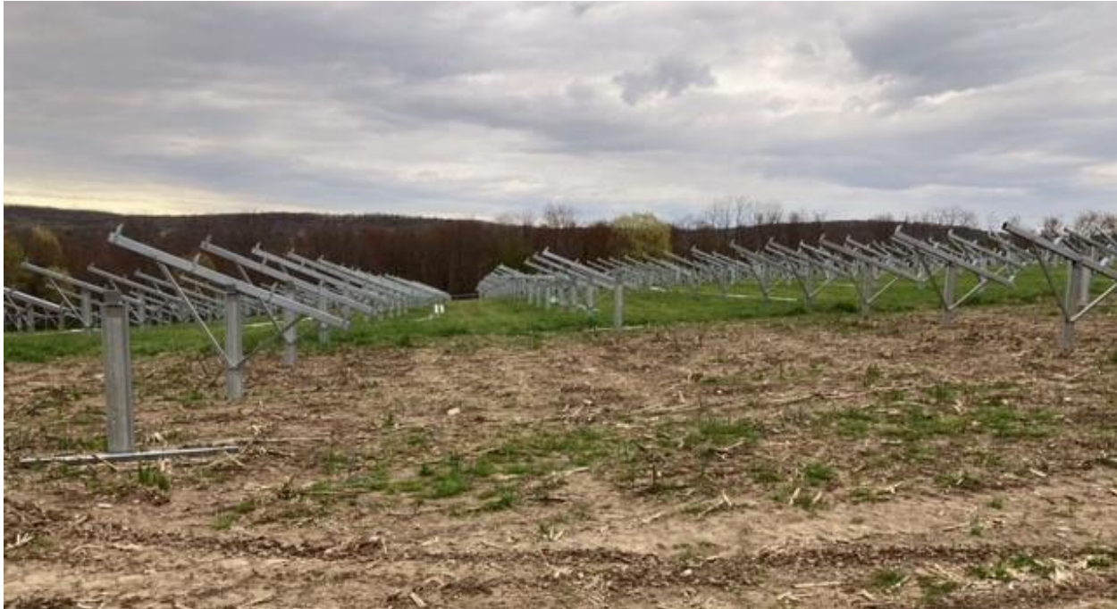
A solar generating system, installed at Baird in 2021
