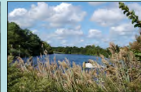
Unhealthy, tidally restricted side of culverts
