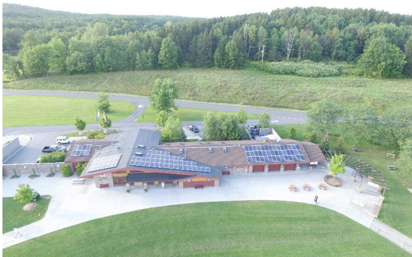
Photovoltaic panels installed on the West Beach Bathhouse roof help offset energy costs at the facility.
