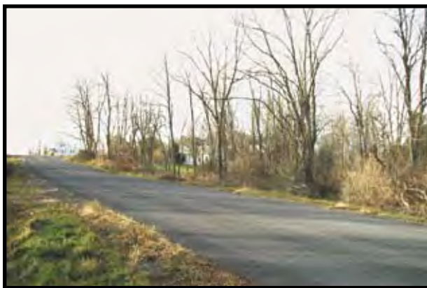
SP 58+900: Trail intersection at Agard Road. Trail crosses road at a cross-slope. Culverts will need to be installed for the trail crossing on both sides of the road.
