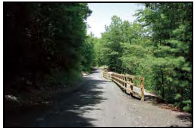
Safety railing, as illustrated in this photo, can also serve to discourage trail users from leaving the corridor and trespassing on adjacent private property. This installation is on the Catharine Valley Trail in the Finger Lakes State Parks Region.
