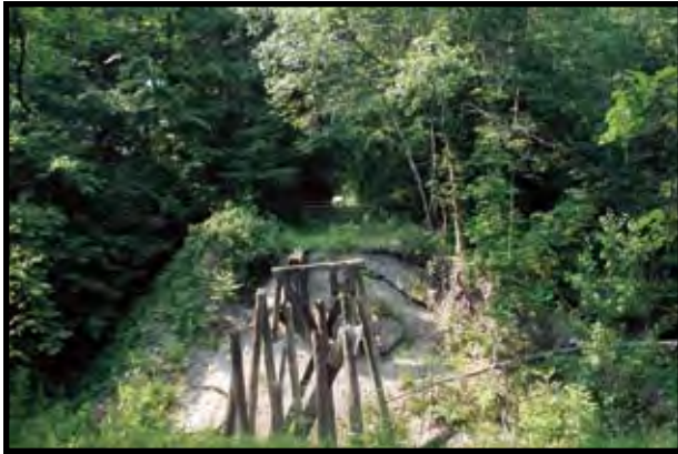
SP 42+250: A new structure for the trail crossing of Glenwood Creek is required. A bridge unit could allow the old trestle-support timbers to be left in place for an interpretive opportunity.
