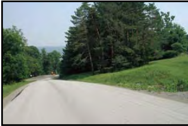
SP 43+700: Trail crossing of Perry City Road. View downslope to N.Y.S. Route 89. Visibility is good in both directions.
