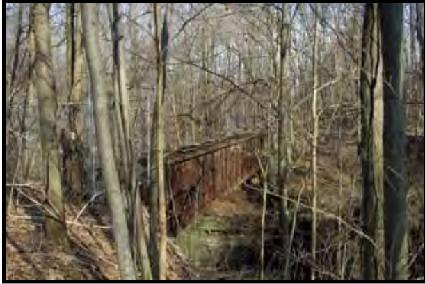
SP 55+100: View, looking south, of the existing railroad bridge over Willow Creek. Redecking and safety railing are needed to put the structure in use for the trail.
