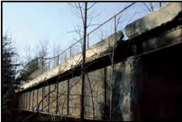
SP 67+200: Existing railroad bridge over Taughannock Creek gorge. The bridge is currently part of the state park’s rim trail system. Upgrades to the structure will be needed.
