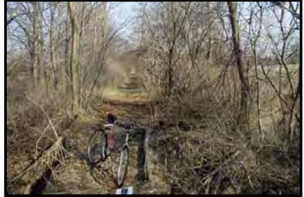
SP 51+700: The lack of maintenance on the drainage structures/system along the abandoned railroad has resulted in several of them failing. Repair and replacement will be needed on many.
