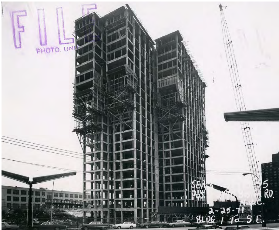
Figure 9: View of the apartment building, looking south, while under construction, February 1971. (NYCHA)
