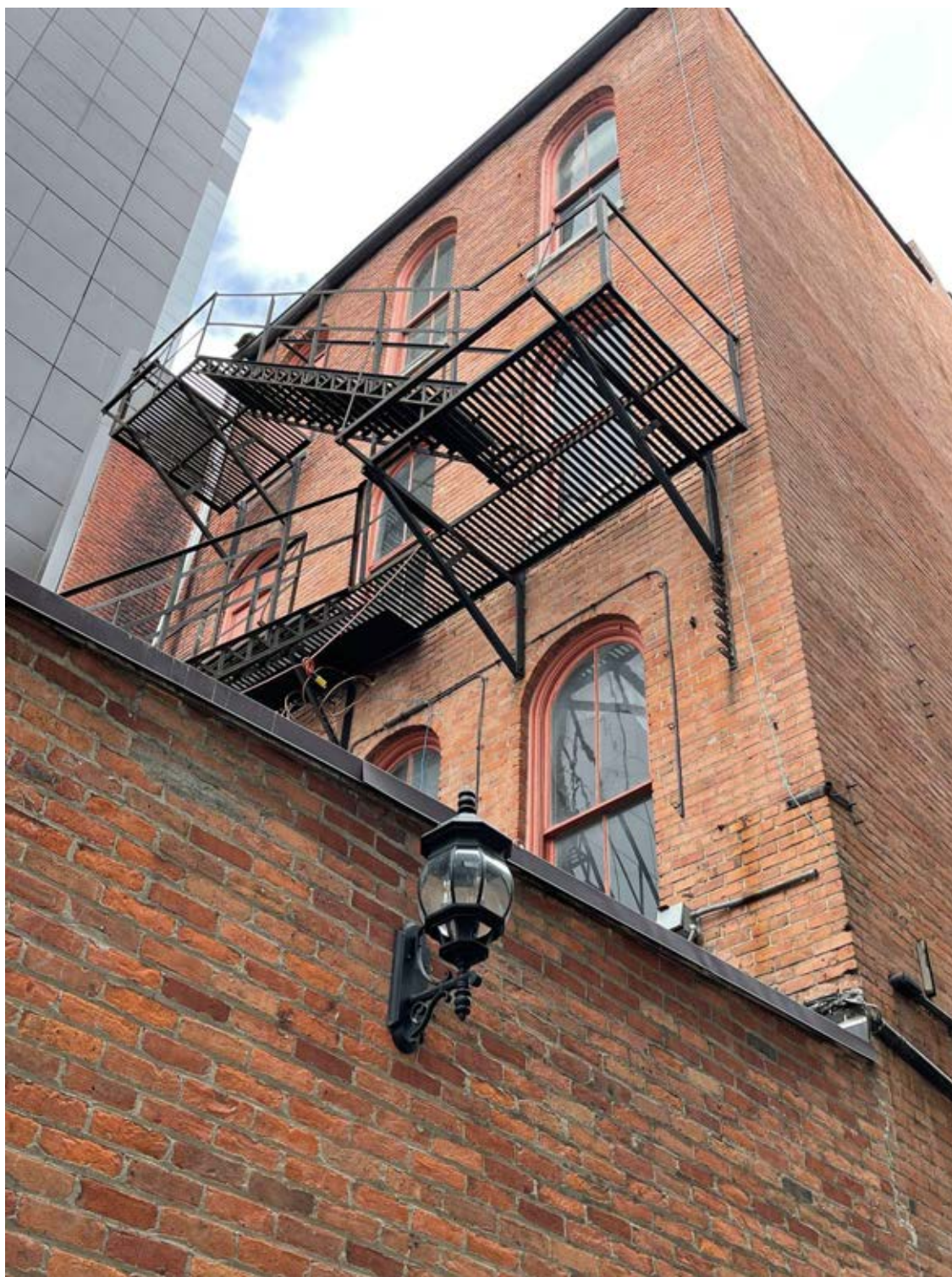
Figure 2.5. South elevation view of 143 East State Street, looking northwest. Photo by Jeff Iovannone, March 8, 2022.
