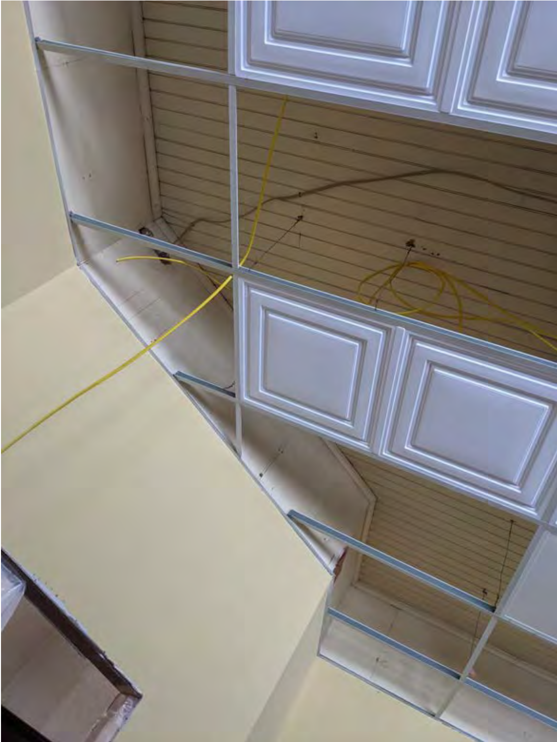
0027 of 0028: Original wood tongue and groove ceiling remains above new drop ceiling, looking up from the first-floor landing.
