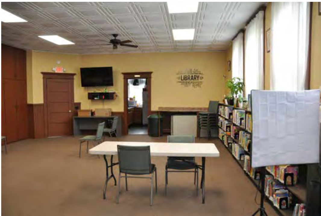
0016 of 0028: East classroom/community room with new door to foyer and doorway to kitchen, looking north.
