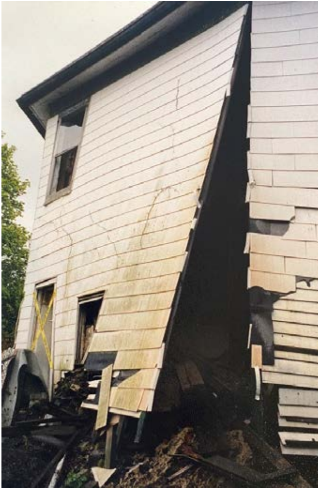
Fig.7: Photograph of house in 2002 showing collapsed section of grout wall. Photo by Jonathon Hallam.
