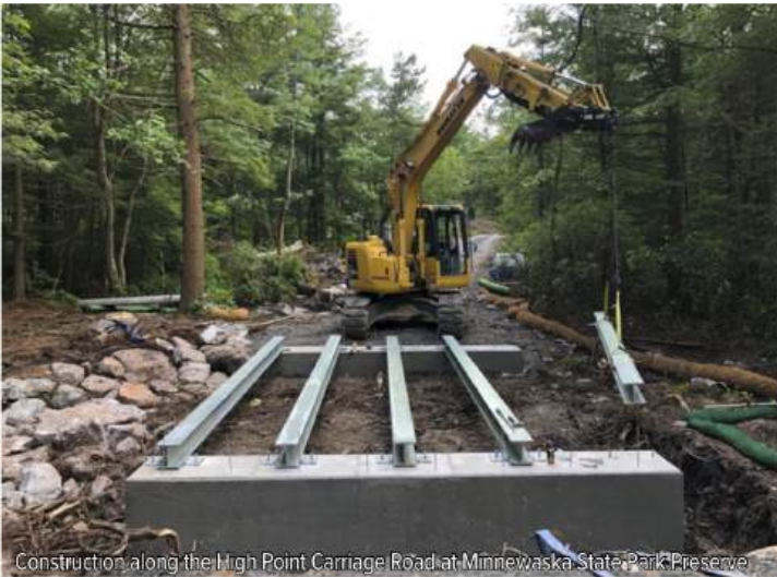
Construction along the High Point Carriage Road at Minnewaska State Park Preserve
